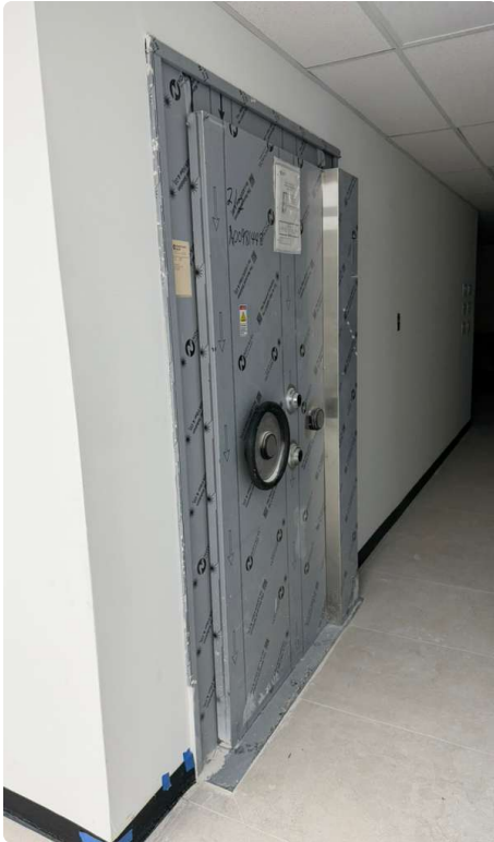
One of 2 walk-in vaults
